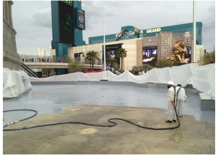
At the New York-New York in Las Vegas, a crew applies VersaFlex's FSS 45DC polyurea basecoat to the reflecting-pool feature. This follows application of a modified polyurethane primer.
