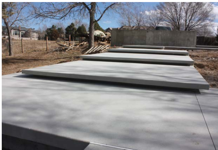
Although the concrete work is done, it doesn't show at its best because the surroundings look rough and shadows detract from the even tone of the concrete.
