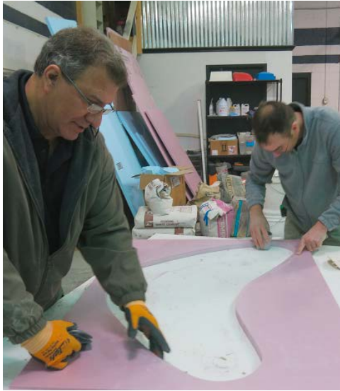
Foam can be used to create a curved table top form. The concrete will be cast inside the hole in the foam.
