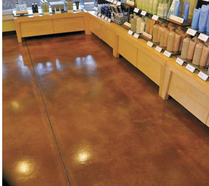
This floor at the Aveda Salon and Spa in St. Petersburg, Florida, was microtopped with Increte's Level Top SP, acid stained with Stain-Crete and finished with a water-based urethane. Work was done by Brian Elsinger with Unique Concrete, formerly based in Tampa and currently in Sioux Falls, South Dakota.
