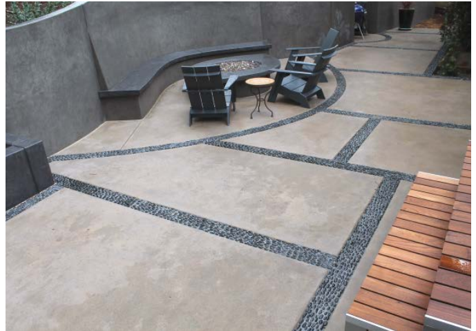
Dorsal fin bands are another creative way to use an unorthodox type of aggregate. For these bands, or veins, 2-inch flat Mexican black pebbles are turned on their side to resemble a fin. Installation is painstaking — one at a time. The fins create an impression of fish swimming upstream.
