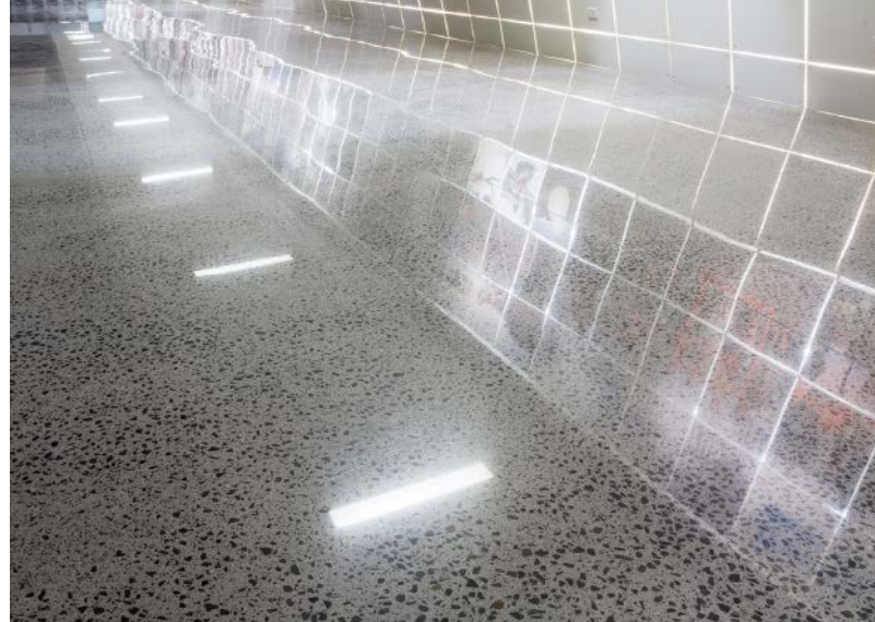
The floor seen here was created with the HTC Superfloor system which produced a highly refined surface with a high-gloss value and above-average DOI. Specification guidelines to fully embrace DOI are in the development stage.
