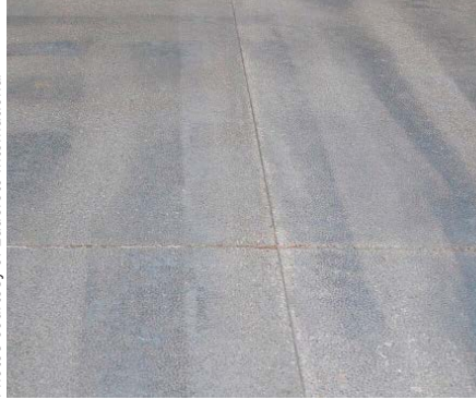
Before a coating was applied, this floor was prepared with bush hammer bits.
