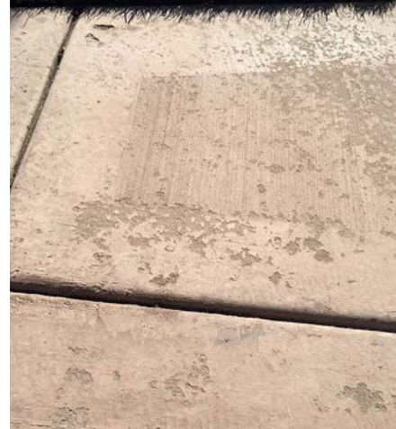
When a concrete slab is overwatered or has had water added during the finishing phase, it is more susceptible to freeze-thaw damage. Leaving concrete unsealed in these conditions can also be detrimental to the overall integrity of the concrete.
