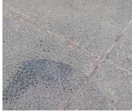
Prior to applying Laticrete's Spartacote Urethane Cement, the surface needs to be mechanically profiled.
