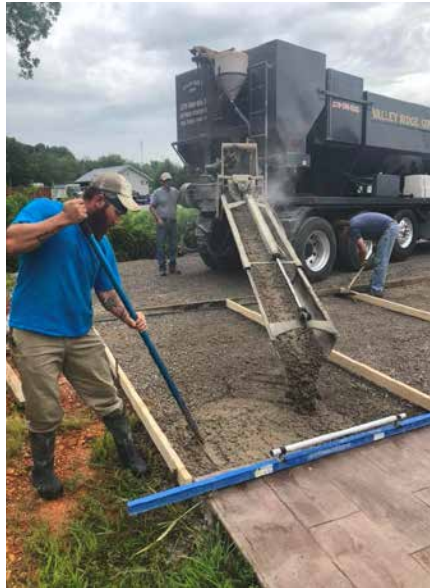
A crew member places colored concrete from a mobile mixer during a training demonstration.
