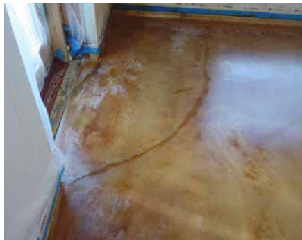
Cold exterior temperatures created a temperature differential on the concrete that led to sealer damage near the door and walls.
