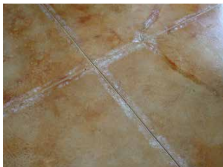
Trapped moisture in saw cuts on a cold slab create moisture haze and efflorescence.
