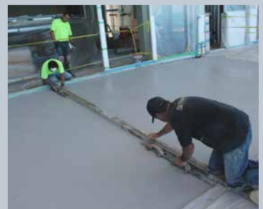
The crew uses chisels and a 2-by-4 as a straight edge to make an initial cut.
