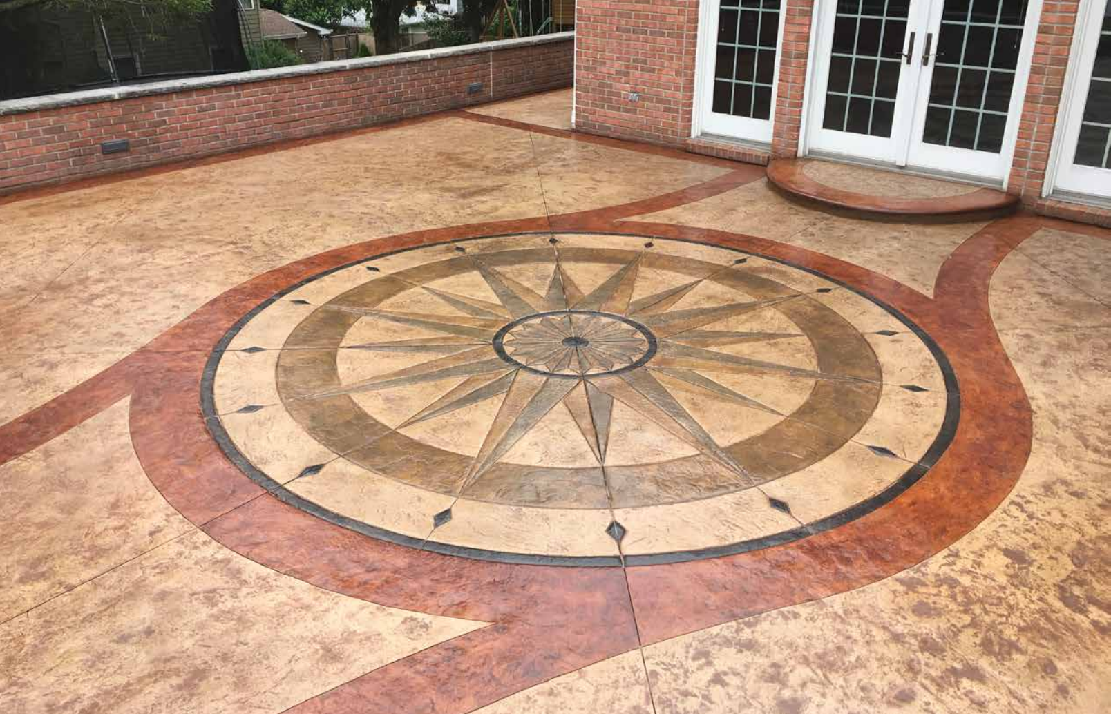
Lack of proper maintenance resulted in the need to strip and recolor this decorative installation. Sealer incompatibility and stain failure figured in the demise of the decorative treatments ( photo below ). The restoration result is pictured above.
