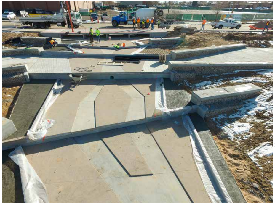
A new drainage structure at 38th and Holly in Denver is being installed for SEMA Construction. The project uses Grasscrete, exposed aggregate, stamped concrete, broom-finished concrete and stain in an innovative design dreamed up by the folks at The Art of Concrete and the landscape architects.
