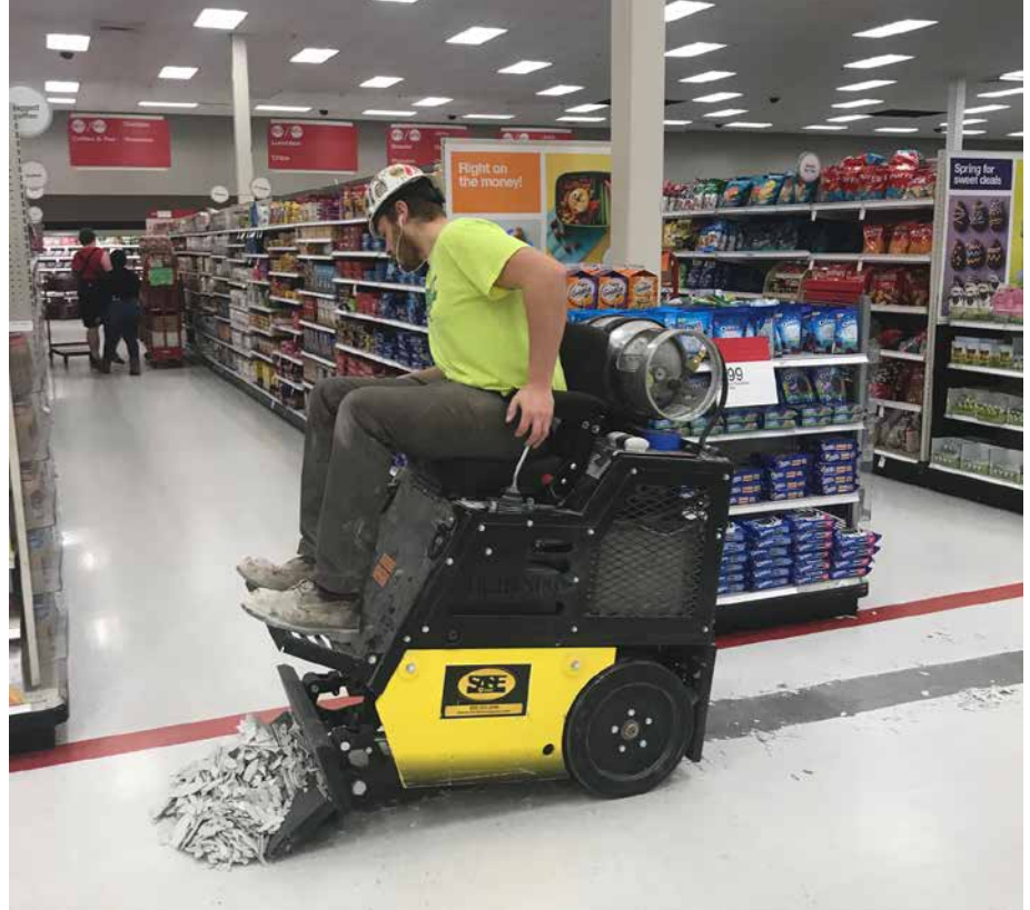
During a renovation on a big-box store that remains open for business, it's typical for a demolition crew to work in one part of the store while polishing crews work in others.
