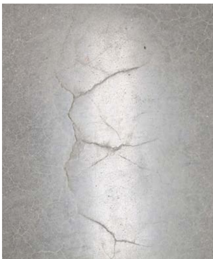
If you look closely, you can see the curvature of the concrete that's a blister that hasn't broken yet.
