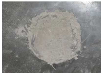
Trapped air can form blisters that will almost always result in spherical-shaped delaminations.
