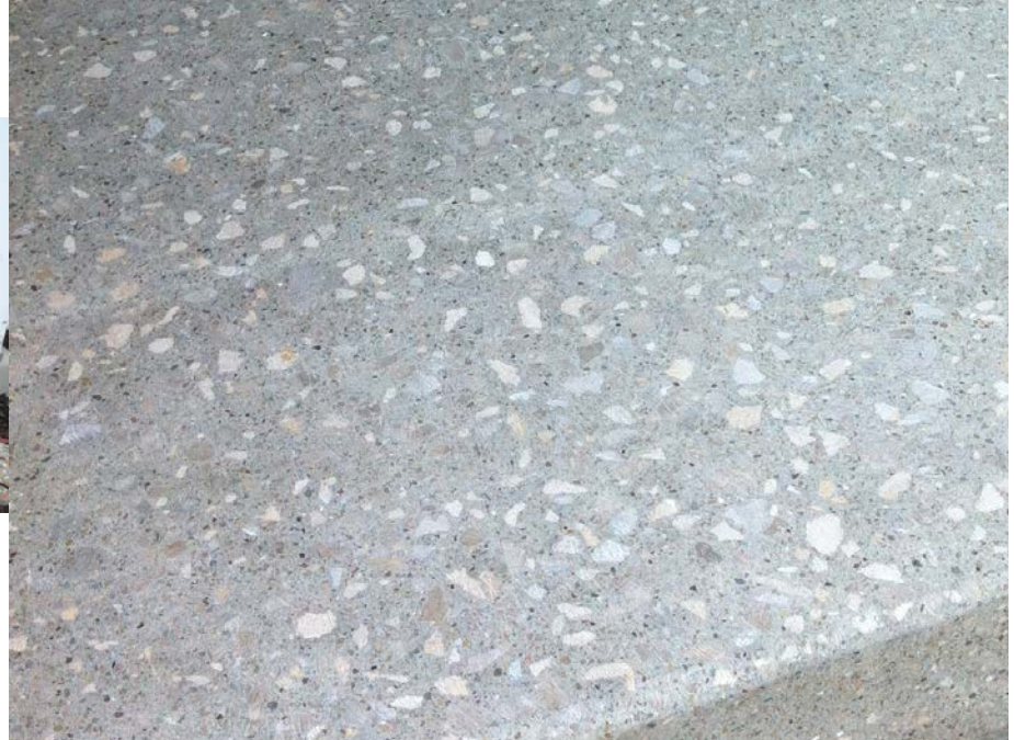
If a slab is in good shape except for the surface, Concrete Contracting Solutions favors a grind-and-seal approach to remedy the problem.
