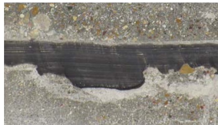
Shaving joints too soon or shaving joints that are wider than the manufacturer's tolerances will leave chatter marks and odd scrapes along the joint that easily stain.
