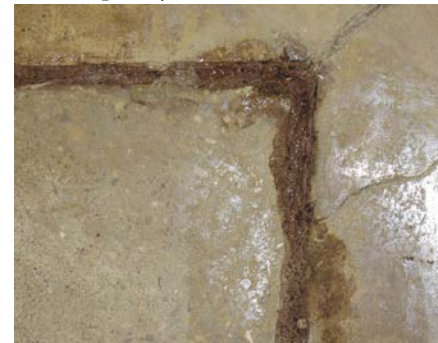
If a joint hasn't had enough time to dry before it's filled, the polyurea will bubble and fizz and never harden properly.
