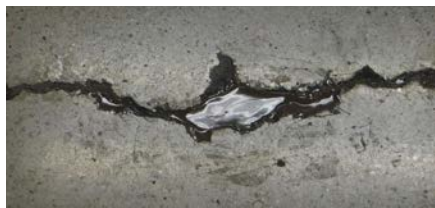
Underfilling a crack creates a maintenance and safety issue.
