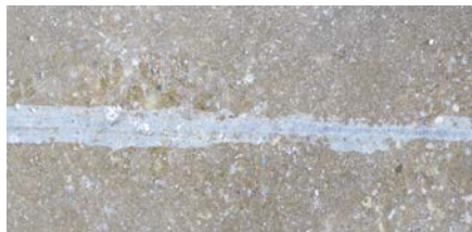
If floors aren't properly cleaned before they're repaired, the residue left behind will soak into pores and leave a pattern that remains even after the floor has been shaved.
