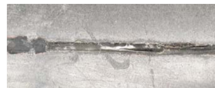
When a repair is underfilled, it can't be ground smooth and will stand out on the floor.
