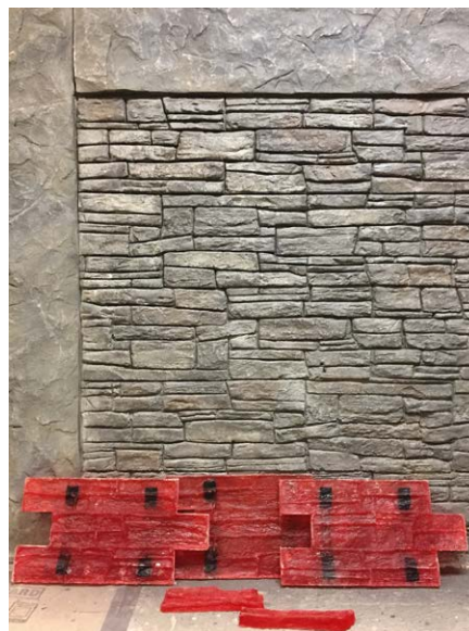
Picture 3: Seen here is a concrete overlay mix applied to a wall and stamped but not colored.
