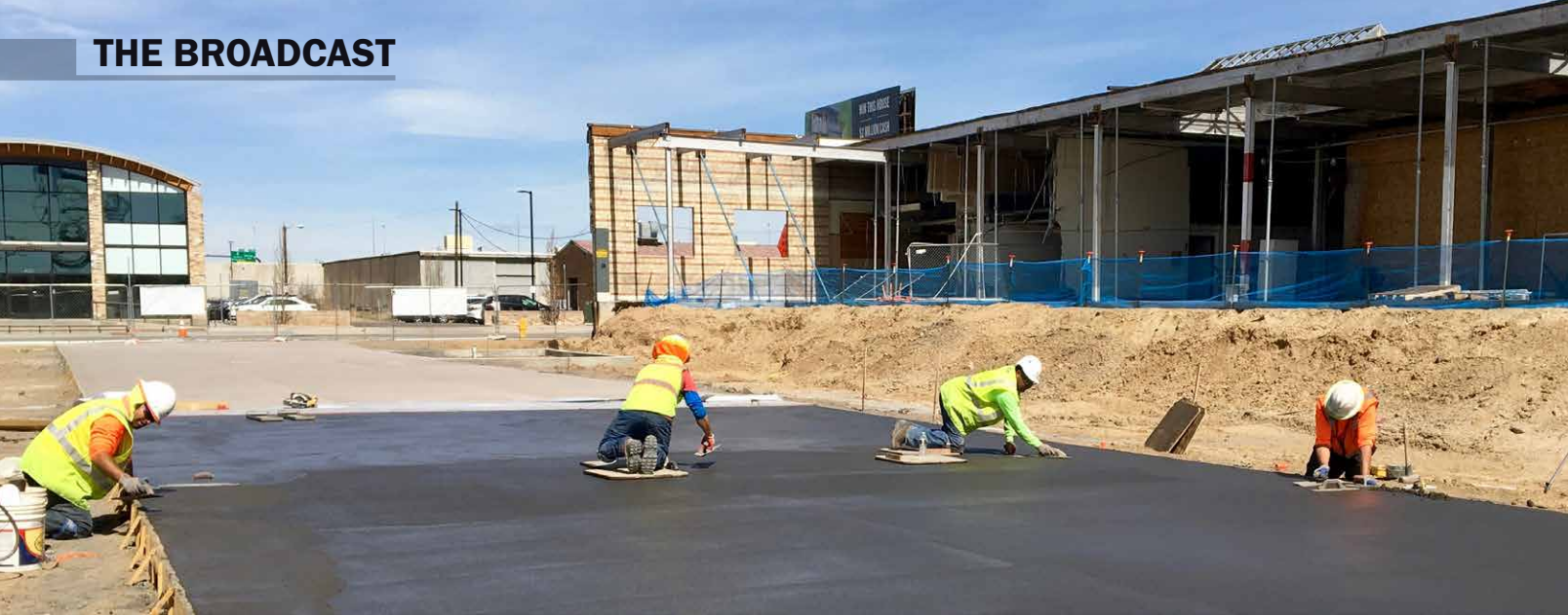
Safety is scrutinized more closely in a commercial project than with a residential job, and organization is paramount to help with its success. Photos courtesy of The Art of Concrete LLC
