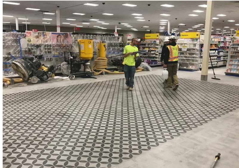
After the Tribeca stencil was stained and removed, the crew applies a densifying sealer.
