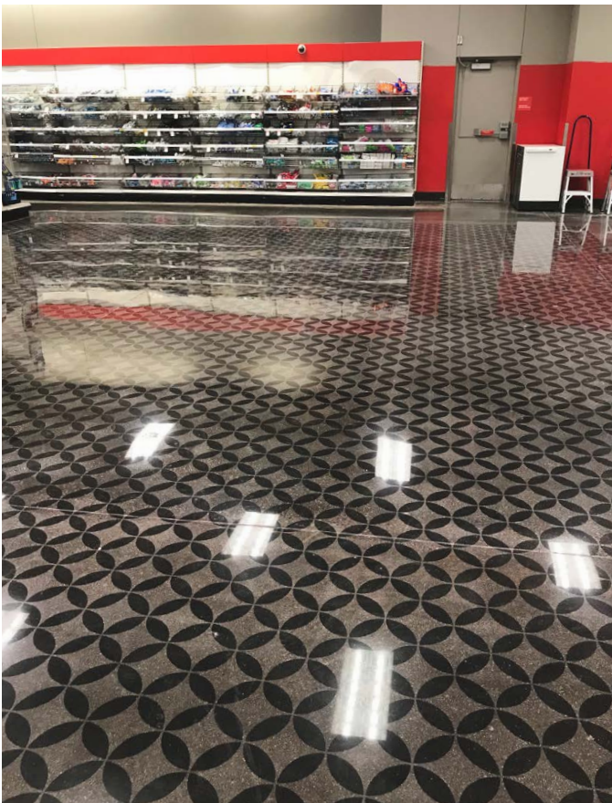
After the Tribeca pattern was successfully stenciled, stain guard was applied and the floor was burnished.
