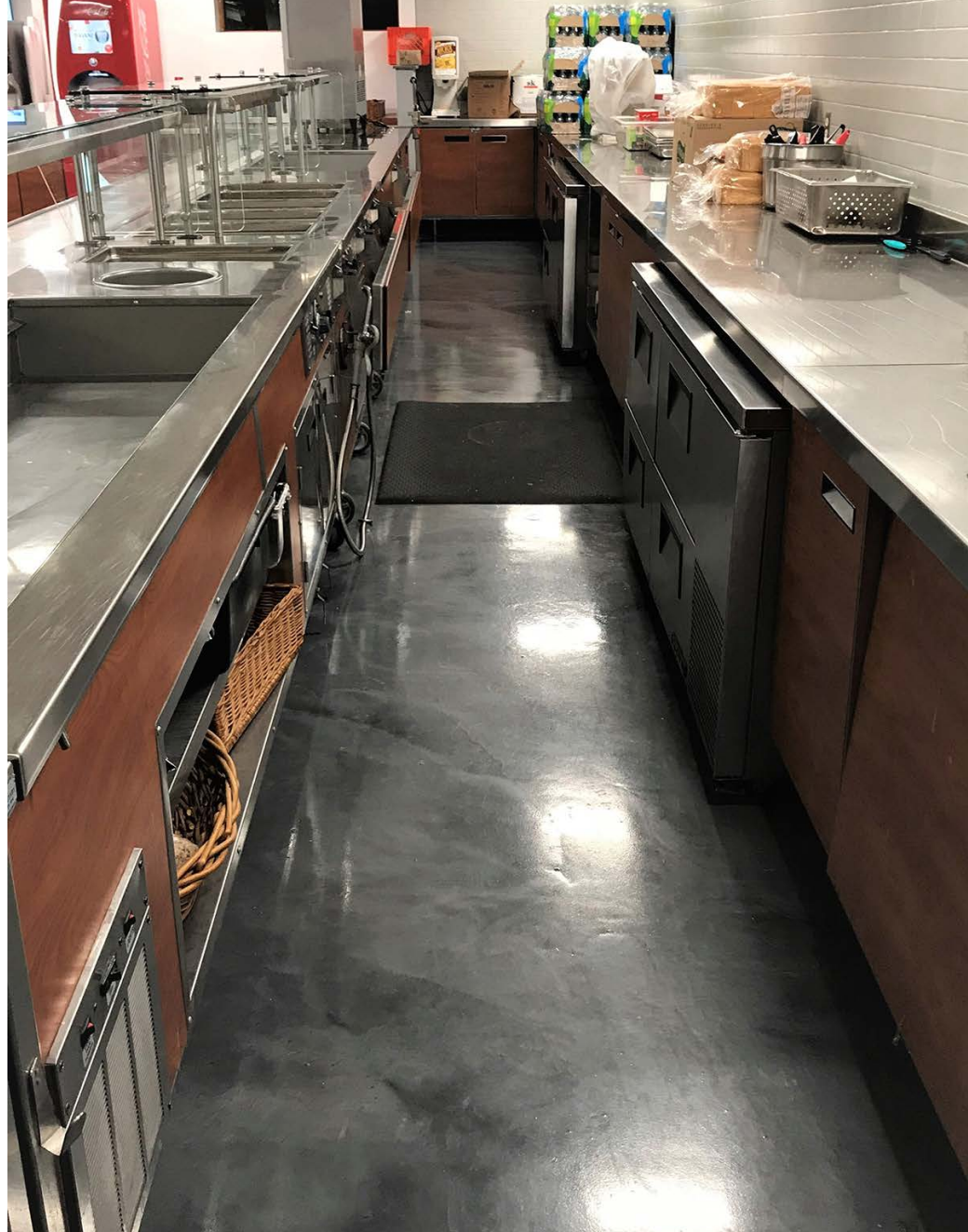
Seman Flooring only had a two-day window to remove the existing floor coating and install a new polyaspartic floor system in the employee café at Nemaocolin Woodlands, a five-star resort in the Laurel Highlands of Southwestern Pennsylvania.
